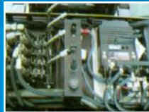
Double controllers with CANbus communication to oil tube and wire
